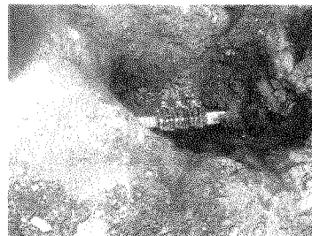
Leak on Chimney Cyn Rd
