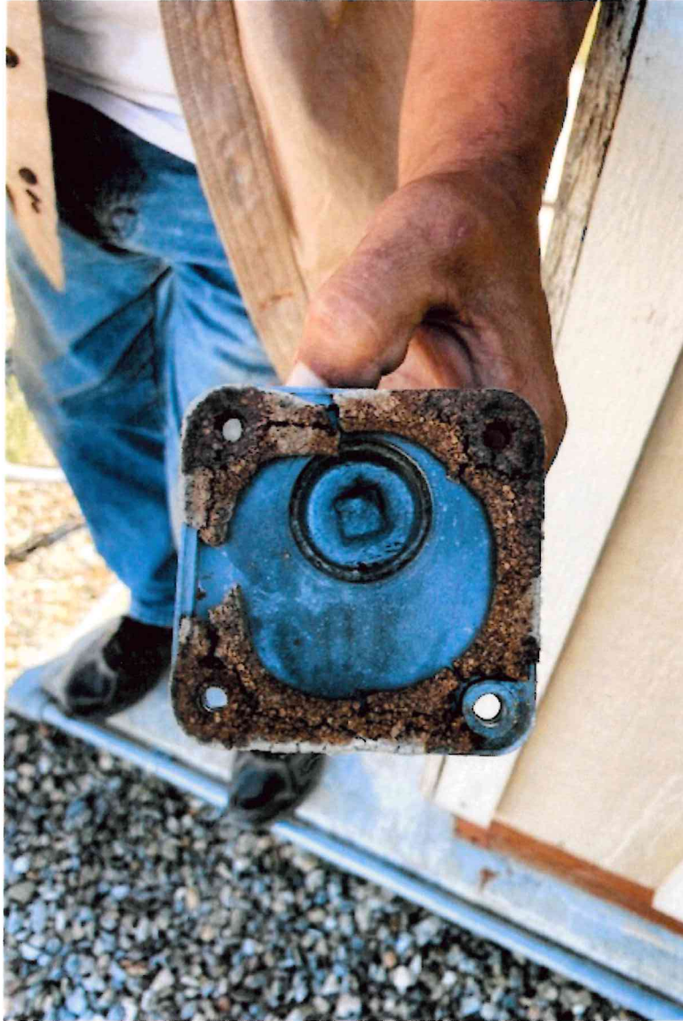
Leban Well Electrical Box Gasket
