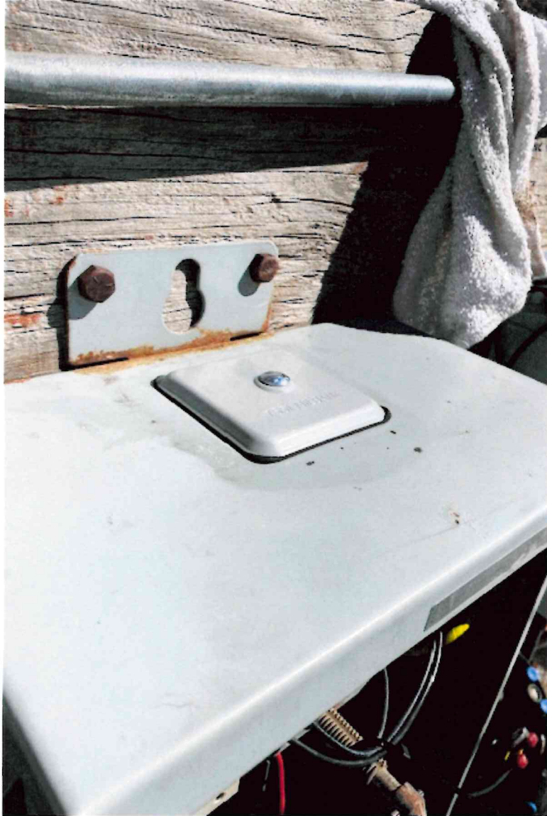
Lebec Well Electrical Box
